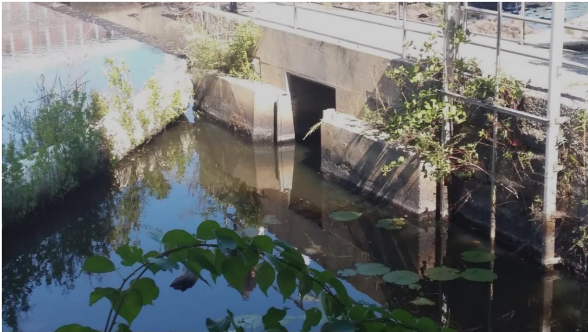
Photograph 32 – Low-level outlet gate and Denil fishway exit looking downstream from right riverbank
