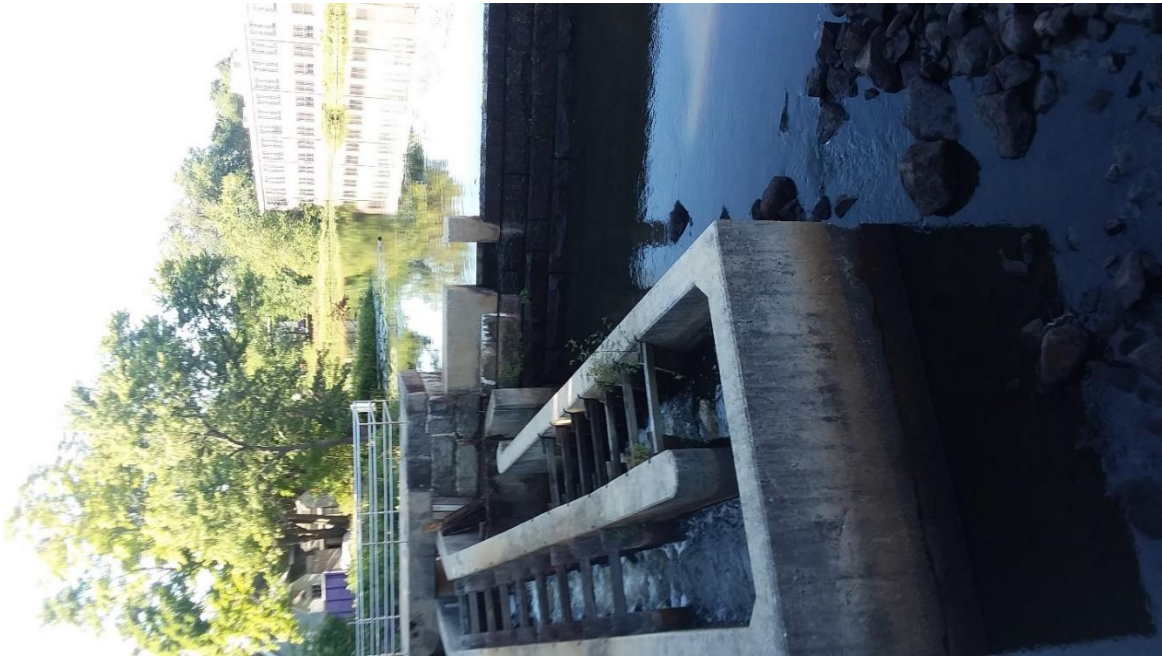
Photograph 25 – Fishway attraction flow outlet in center of photograph on dam crest adjacent to fishway
