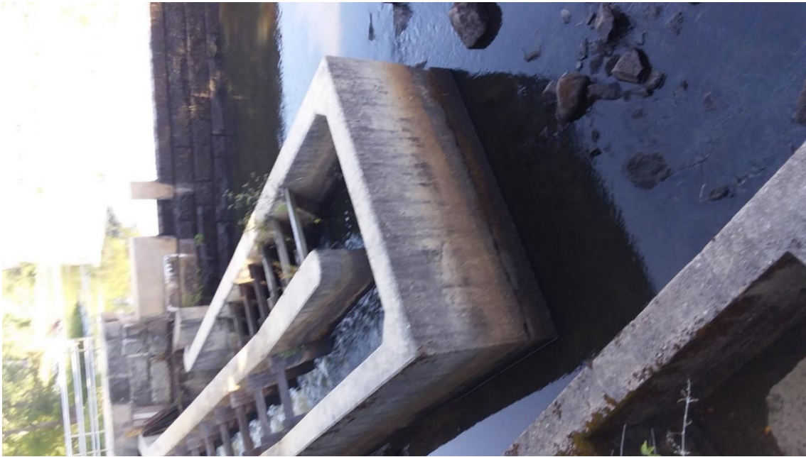
Photograph 21 – Wall and base slab construction joint concrete erosion at fishway turning pool
