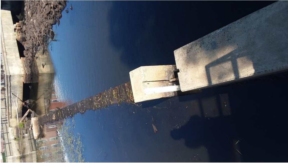
Photograph 27 – Dam crest and fishway attraction flow outlet with staff gage looking from fishway exit
