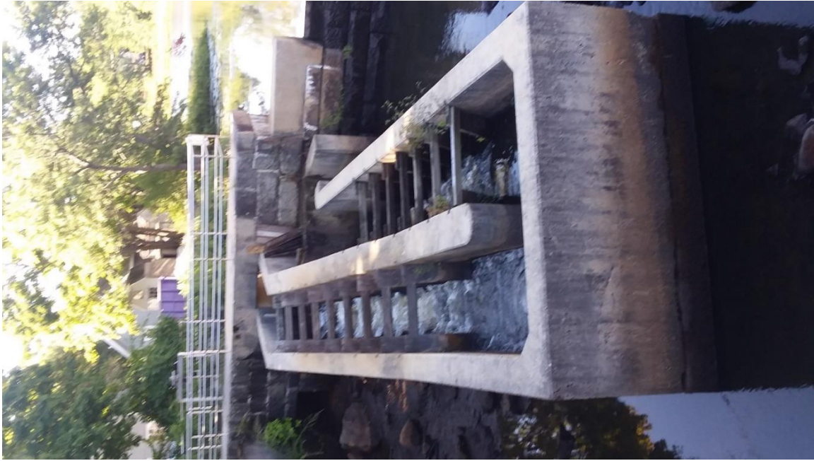
Photograph 23 – Low-level outlet on left, Denil Fishway, and fishway attraction flow outlet on right
