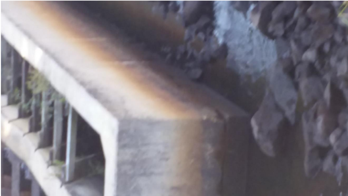
Photograph 18 – Concrete erosion at fishway turning pool wall and footing construction joint
