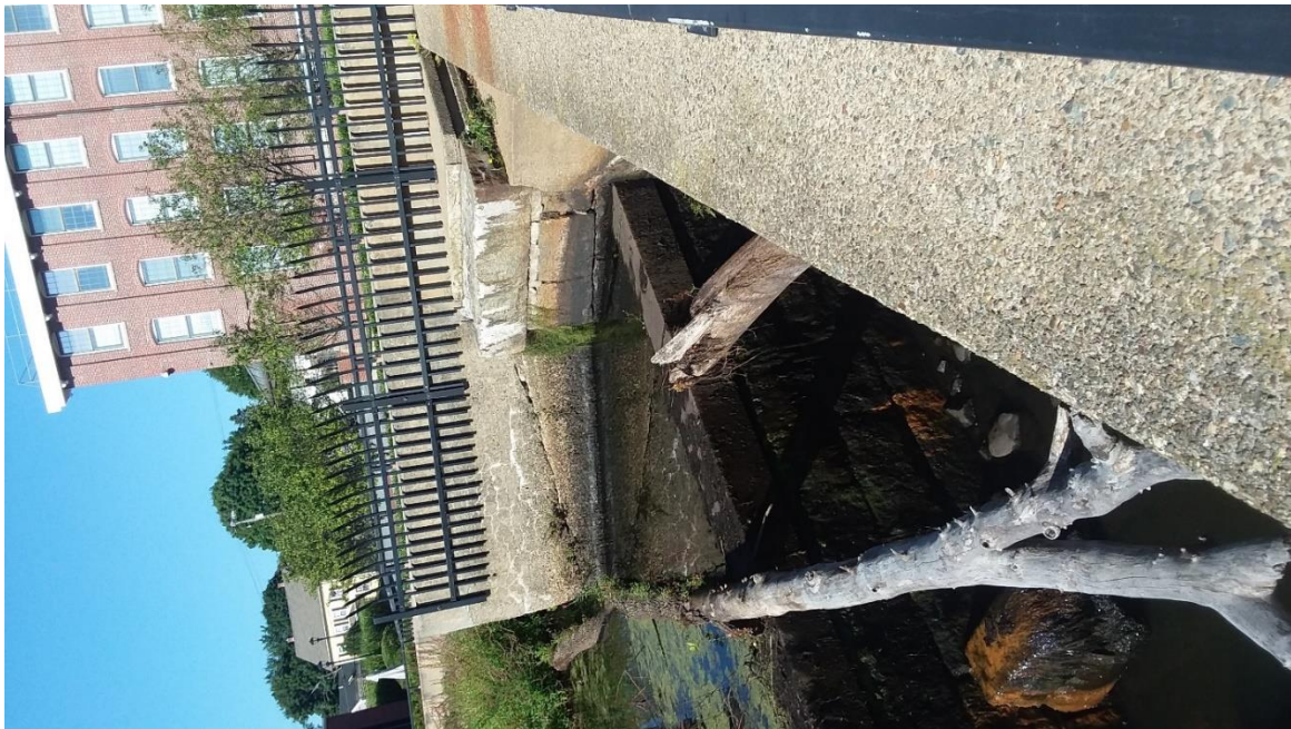
Photograph 16 – Logs on dam crest at left abutment
